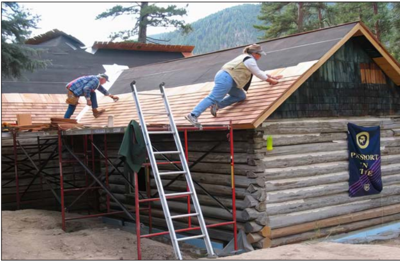
Figure 12. Passport in Time (PIT) volunteers and Forest Service employees re-roofing Morgan-Case in 2003.
